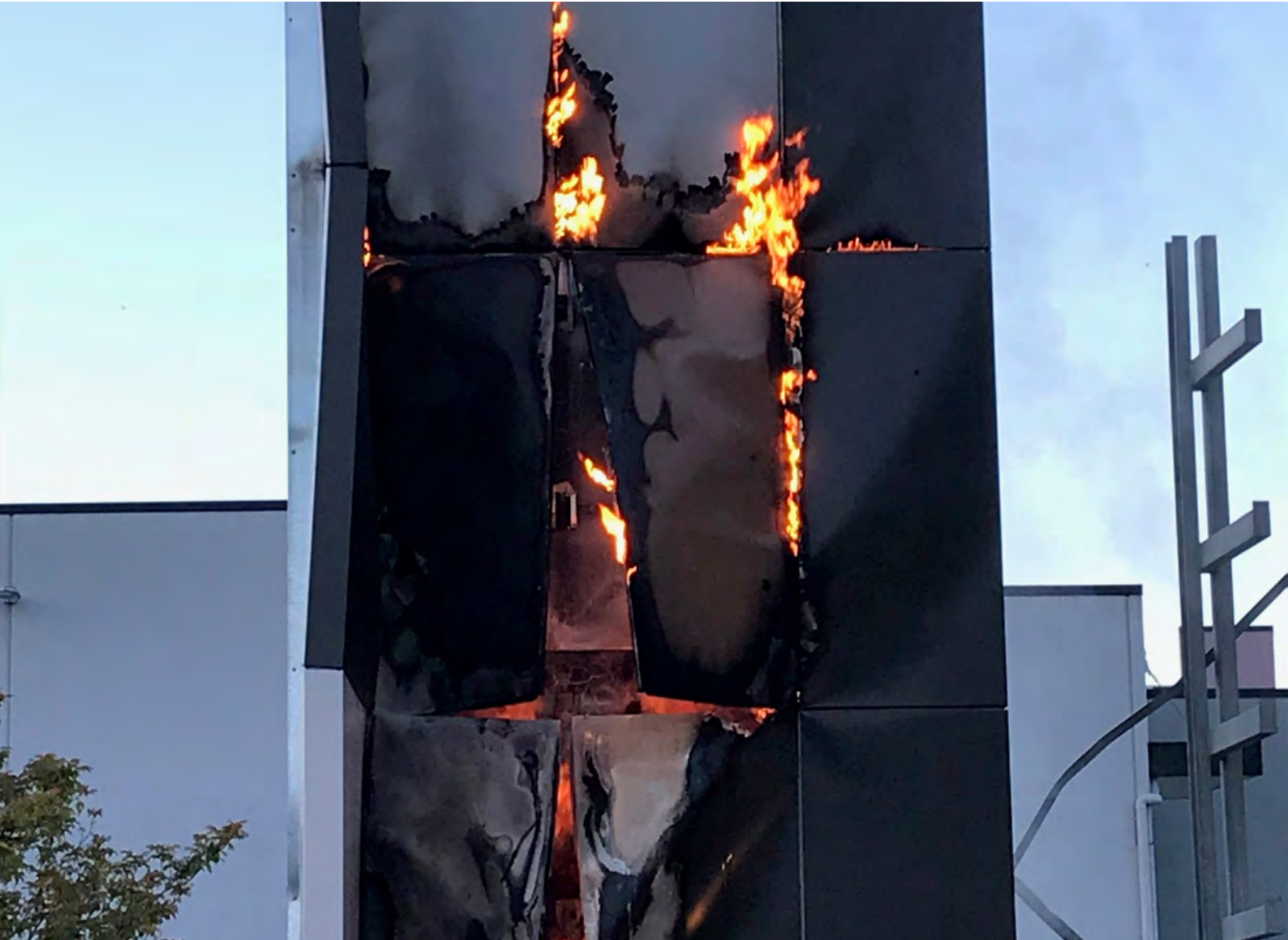
Early grade composite materials are considered highly fire hazardous materials, and have attributed to numerous building fires across the globe.
